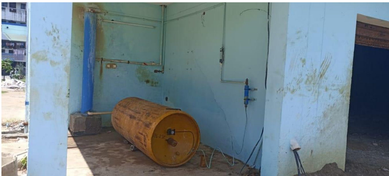
Fig: 7 Chlorine cylinder for chlorination of water (chlorine pumped through the pipes to the filtered water for disinfection)
