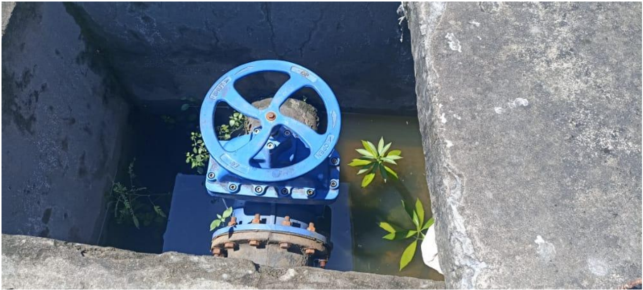
Fig: 8 Valve for pumping filtered water into large storage tanks
